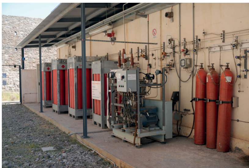
Hydrogen storage and distribution grid
